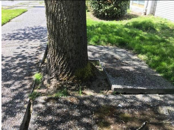
Photo 22: Tree #5105 (Remove), Tulip tree; structural roots pushing up concrete walkway.
