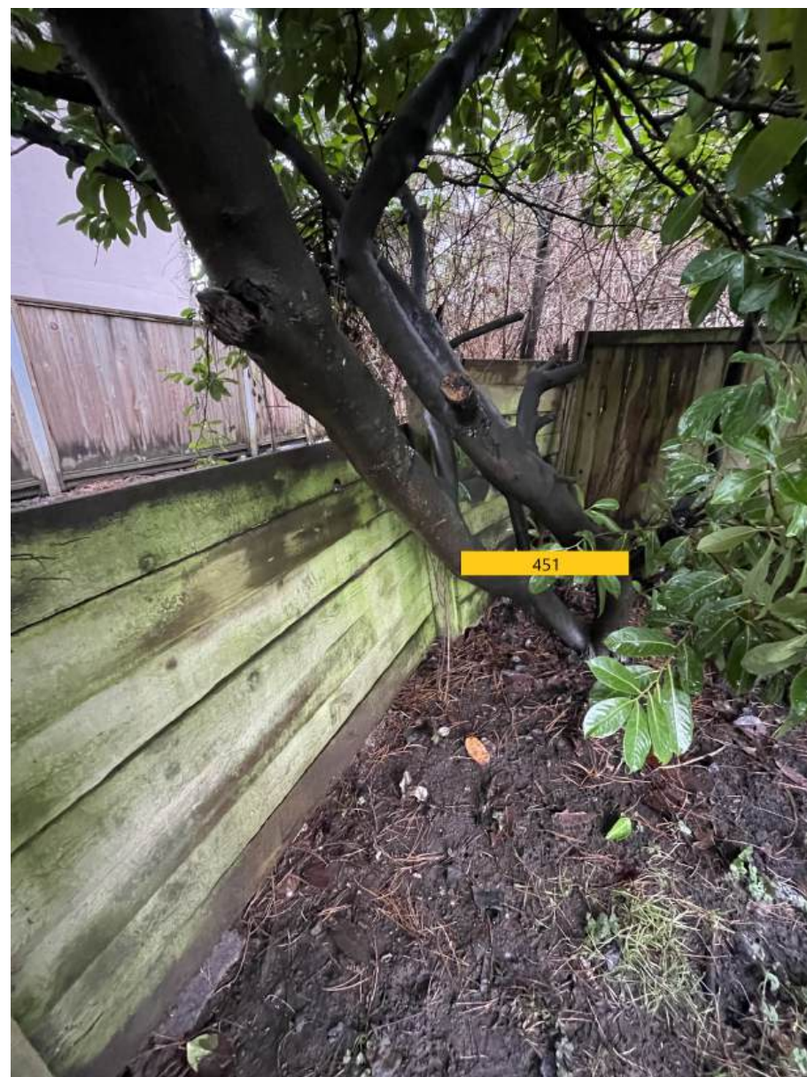
IMAGE 48-Tree base, tree 451- to be removed
